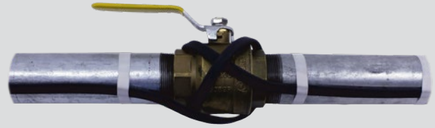
Pipe freeze protection
